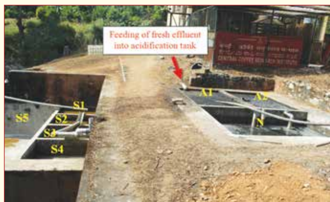
Fig 3 B. A view of new treatment method - Acidification-Neutralization-Sedimentation-cum-Filtration
